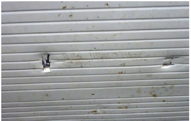
Picture 8 Cargo or forklift truck mast damage to the aluminium ceiling panels.
