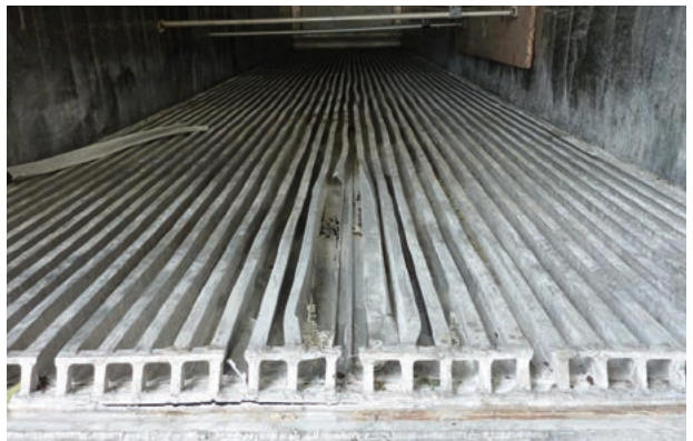
Picture 5 Badly damaged aluminium T Floor showing broken T sections, cracks to the welds which will require major and expensive repairs.
